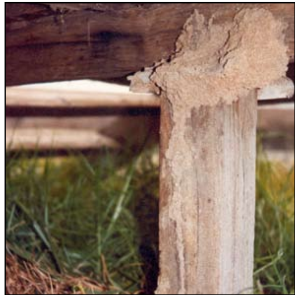
Termite attack on a stump
